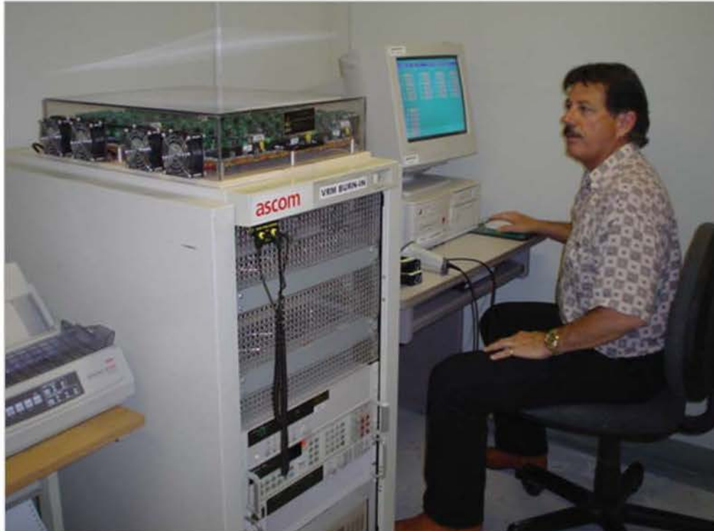
Front view of VRM Burn-In System
