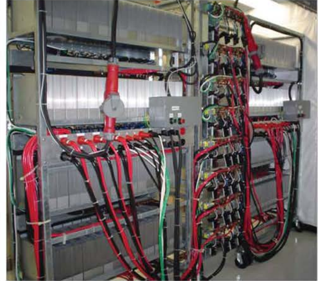
Rear view of Burn-In Cart and Inverters
