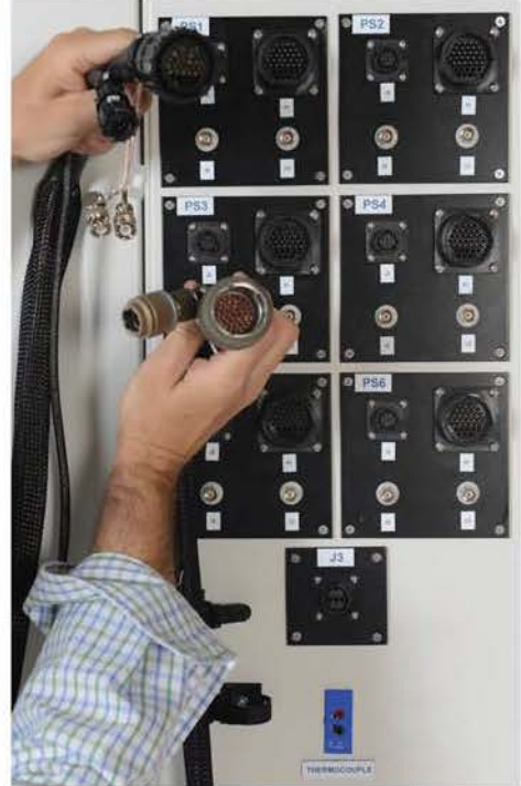
Close-Up of Cable Connections on Rear Panel of System
