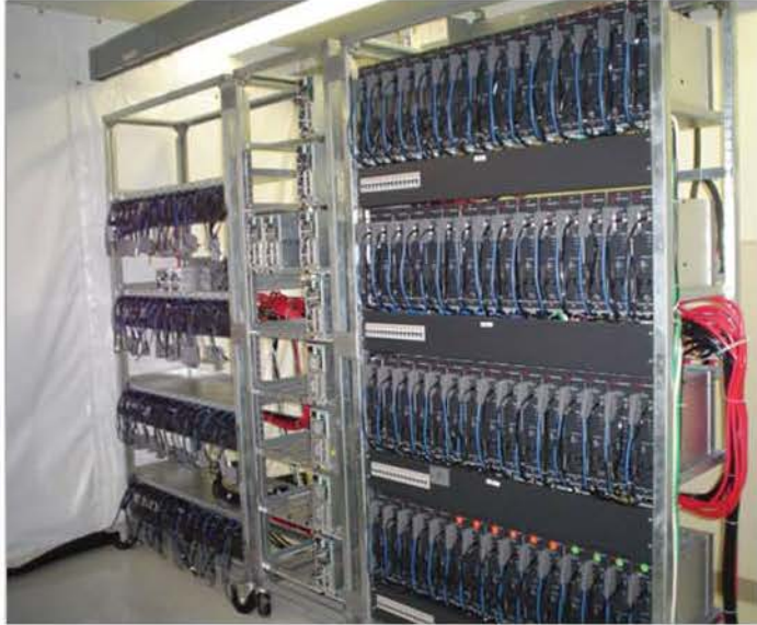
Front view of Burn-In Cart and Inverters
