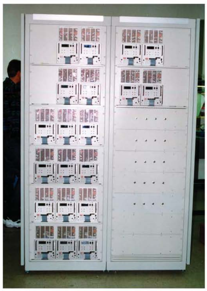
20 DC Power Supplies and fused AC Power Switching Units
