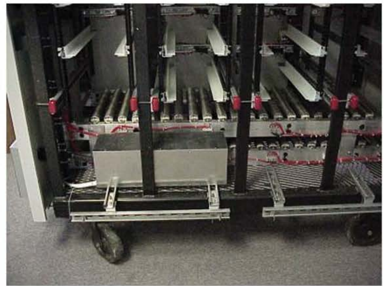
Close-Up of Resistive Loads on bottom of Cart
