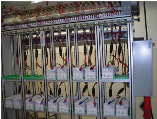
Close-Up of Burn-In Cart with AC Input Power Control Box on the side of the Cart
