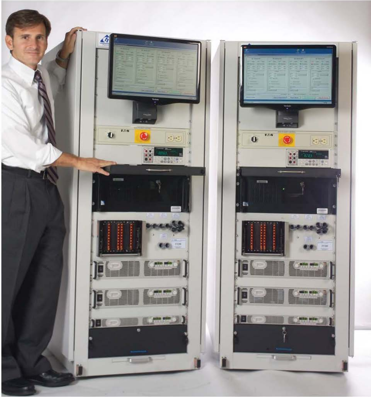
Front view of two DC Monitoring Systems
