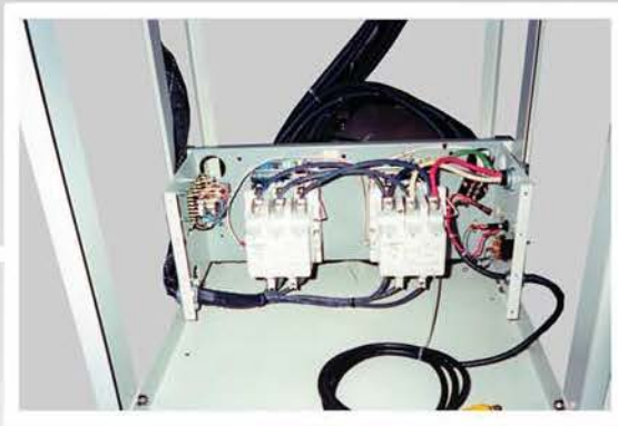
Power Cycling Contactors in Cart
