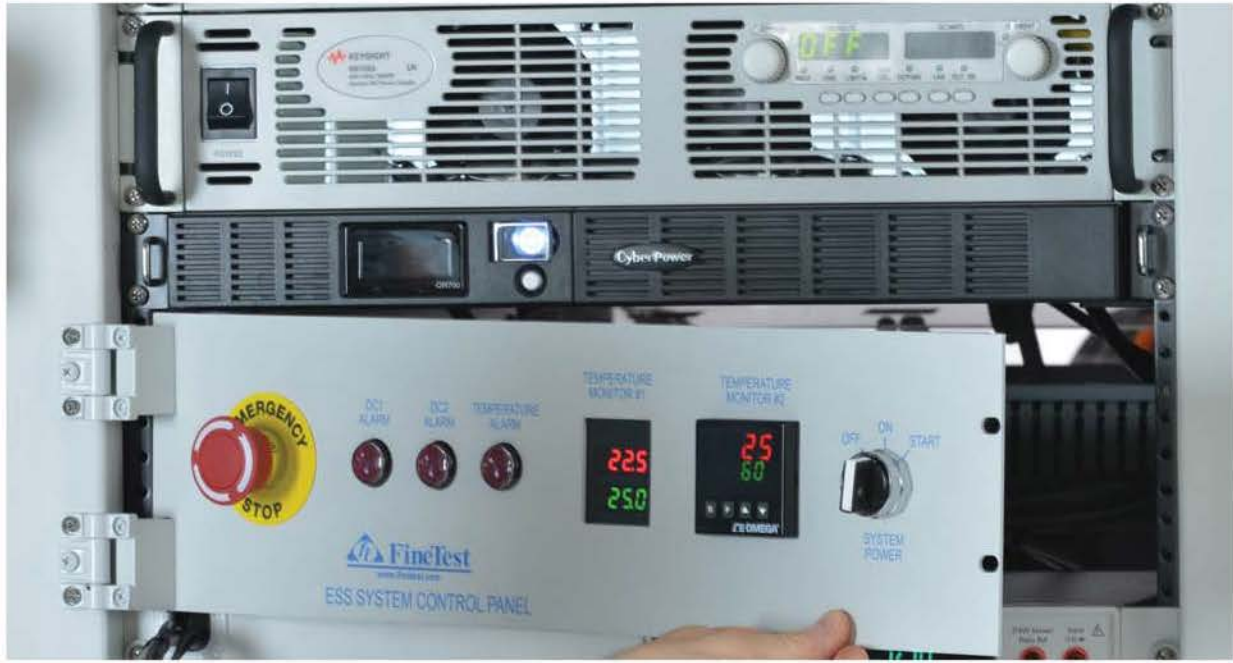
Hinged ESS System Control Panel with Dual DC Input Voltage Monitors and Two Chamber Temperature Alarm Circuits
