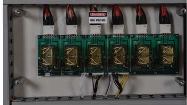
Close-Up of 6 Relays to switch AC Input Voltage On/Off to the UUTs for AC Cycling Tests
