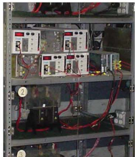
Close-Up of Electronic Loads and Temperature Controlled Chamber with 2 UUTs loaded
